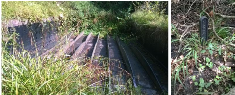
Cast iron aqueduct / NRC marker post in the undergrowth on the old course
